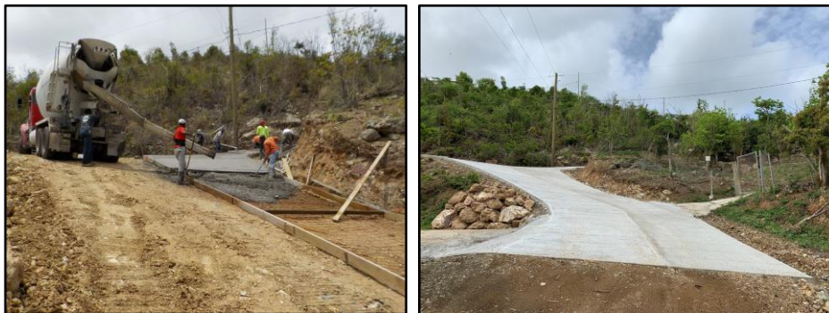
Figure 2-31. Gerda Marsh road stabilization on St. Johns, USVI. Source: Coral Bay Community Council
