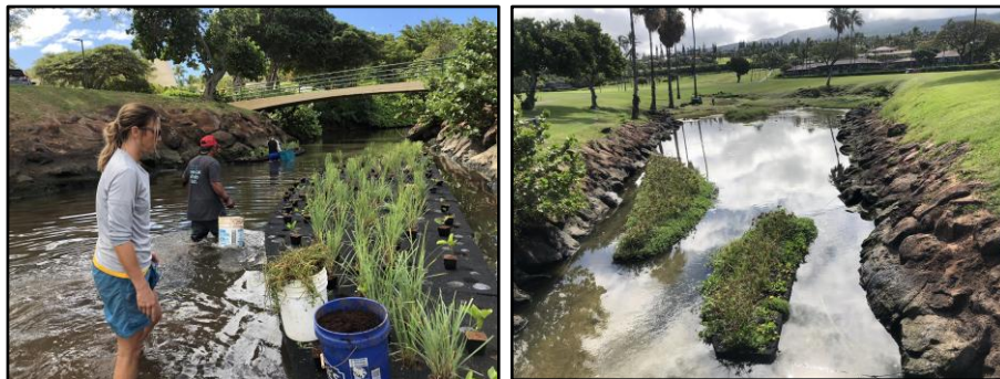
1864 1865 Figure 2-38. Example of an under construction (left) and finished floating wetland (right). Source: West Maui Ridge to Reef
