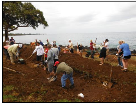
1804 1805 Figure 2-35. Constructing a rain garden in West Maui. Source: West Maui Ridge to Reefs
