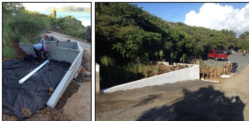
1866 1867 Figure 2-39. Building constructed wetland (left) and finished wetland (right). Source: Protectores de Cuencas
