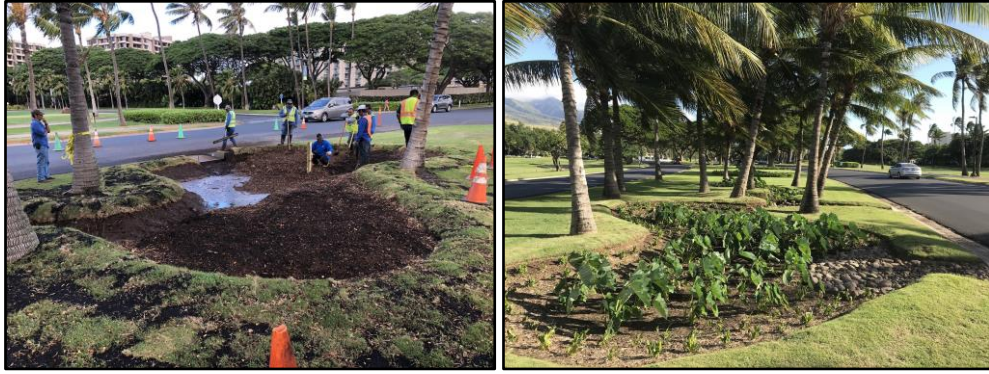
1802 1803 Figure 2-34. Constructing (left) and finished (right) bioretention area in West Maui. Source: West Maui Ridge to Reefs
