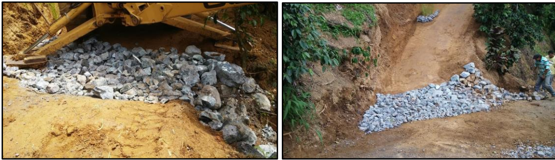
1834 1835 Figure 2-36. An example of swale construction in Puerto Rico. Source: Protectores de Cuencas
