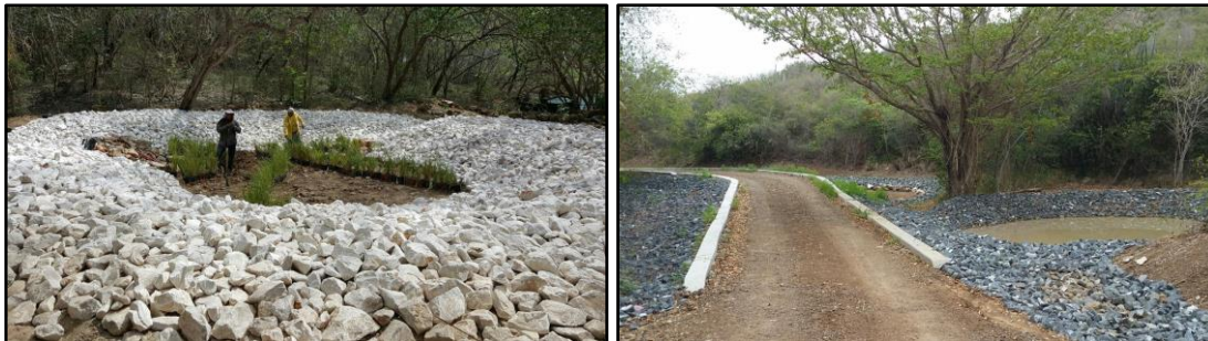
1843 1844 Figure 2-37. Examples of constructed stormwater ponds in Puerto Rico. Source: Protectores de Cuencas
